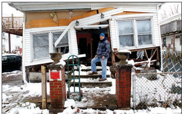
Rudy Mienert, a member of Our Lady of Lourdes Parish in Staten Island, stands outside his destroyed home in the New York borough on Nov. 8. More than a week following the havoc of Hurricane Sandy, residents were struggling to cope with destruction and loss. Special collections were to be taken in all New York archdiocesan parishes over two weekends to help aid in recovery.
