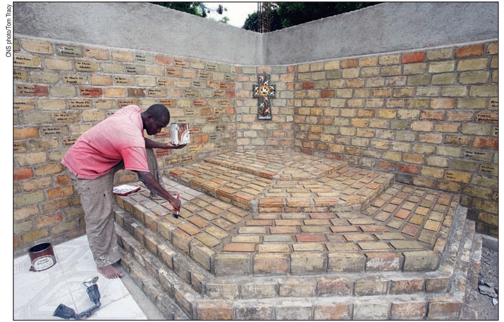
A worker applies a glaze to a new Haiti earthquake monument to remember the deceased clergy, seminarians and parishioners at St. Louis King of France Parish in Port-au-Prince, Haiti. Many people lost their lives when the church collapsed in the Jan. 12 catastrophe.
