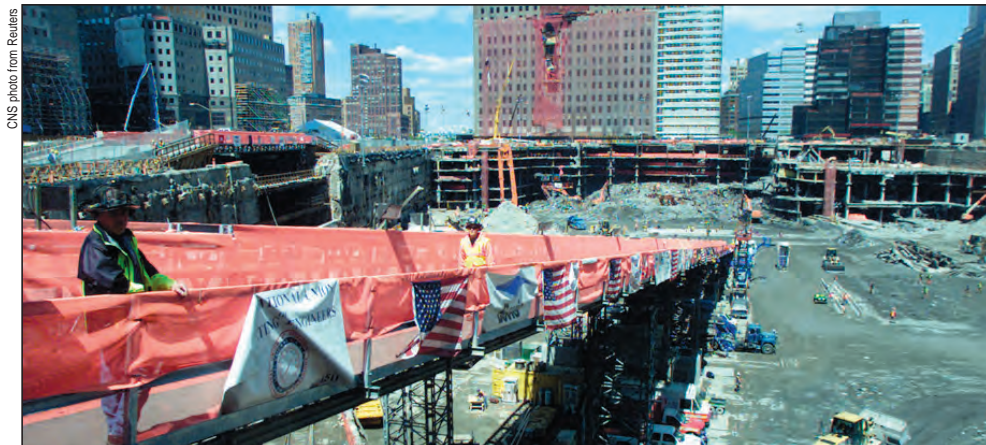
Firemen walk along a construction ramp leading into the World Trade Center disaster area on April 26. Debris removal and recovery work at the site is expected to end by June, nine months after the Sept. 11 terrorist attacks.
