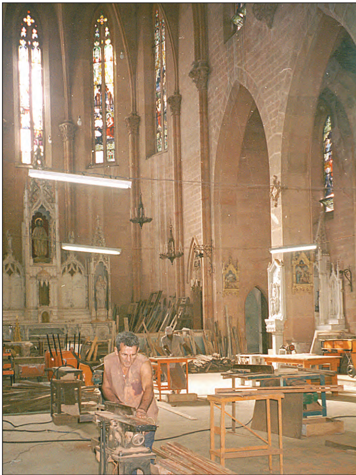
At right, restoration work at the Cathedral of Santa Ana in Camagüey is being completed by volunteer laborers. After Pope John Paul II's visit to Cuba in 1998, the Church received permission from the government to restore some damaged churches.
